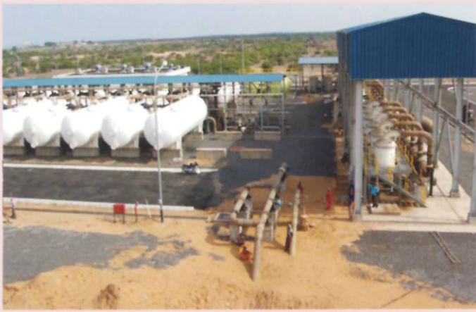
100 MLD desalination Plant - Minjur
